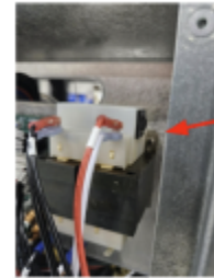
Figure 13a voltage select White Wire position 208V- middle tap 230V -right tap
